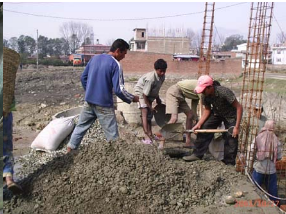
Photo 27: Mixing cement without PPE
