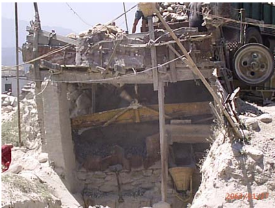
Photo 20: Stone Crusher plant
