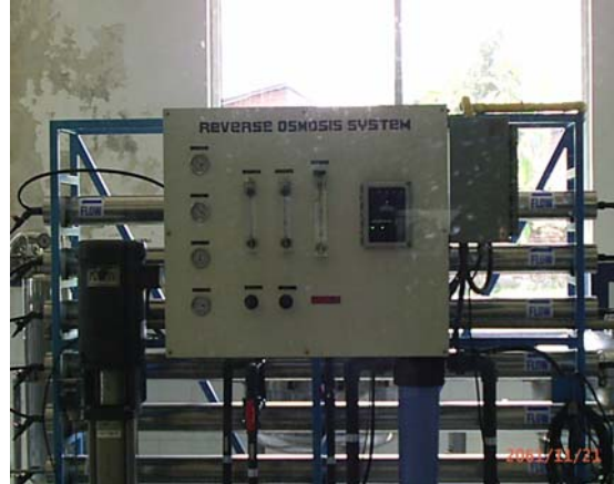
Photo 14: Reverse Osmosis Plant
