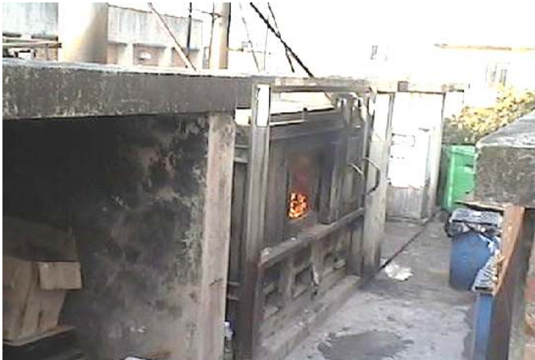
Photo 18: Incinerating of the Infectious Waste at TUTH
