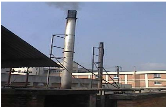
Pic 17: Incinerators at TUTH
