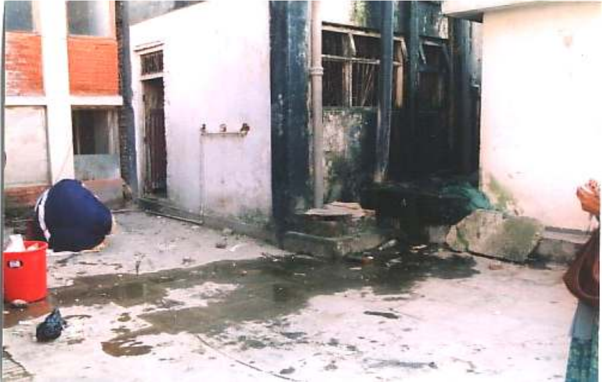
Photo 3: Spillage of wastewater at back of the Bir hospital
