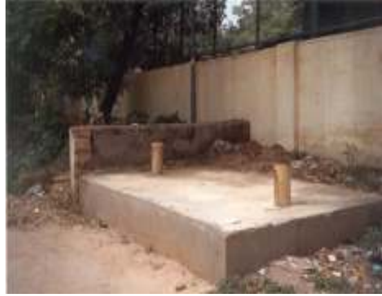
Pic 28 (b) The sharps pit with two openings to ensure even distribution of sharps
