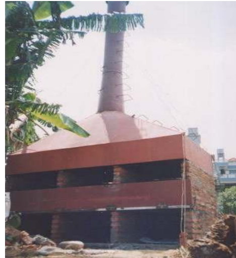
Pic 20: Incinerator of Om hospital
