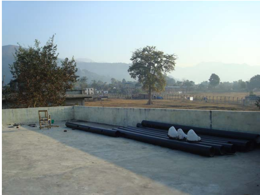
Storage of building materials on the roofs may retain water
