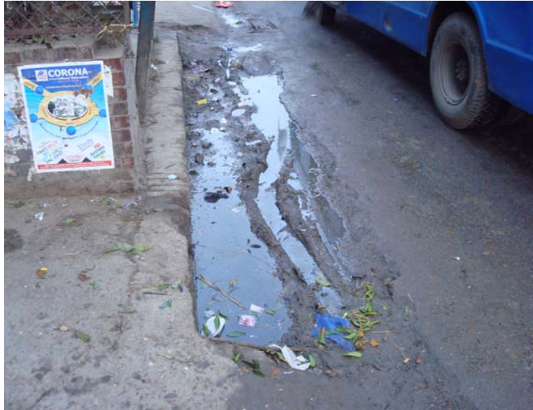
Unpaved and undulated surface with waste water littered
