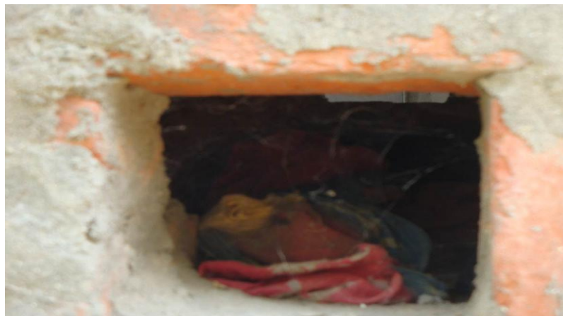
Fig 10: View of pad incinerator at Tikapur
