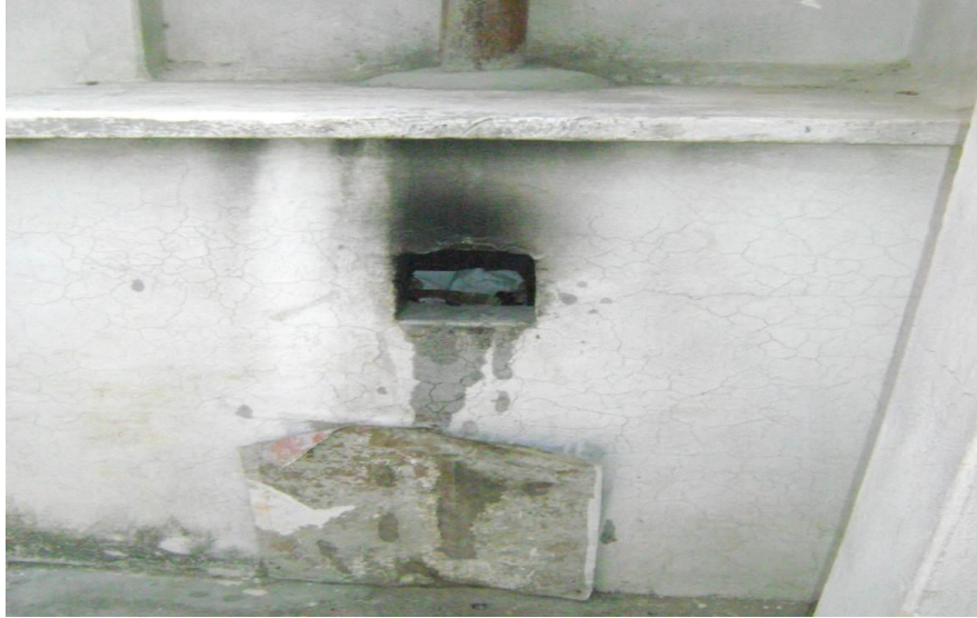
Fig11: View of pad incinerator at Guleria
