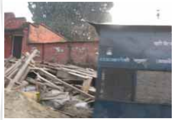
Unclear of Construction Formwork after Buiding Construction
